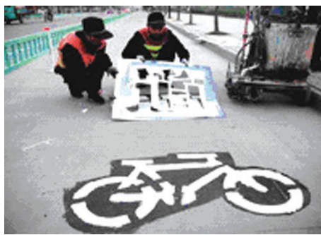
Utility workers paint bicycle lane signs on a road in Chaohu City, Anhui Province.
